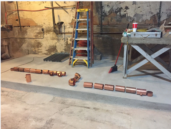
(still a little ways to go on the boiler)
